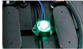
Electrolyte level is OK
